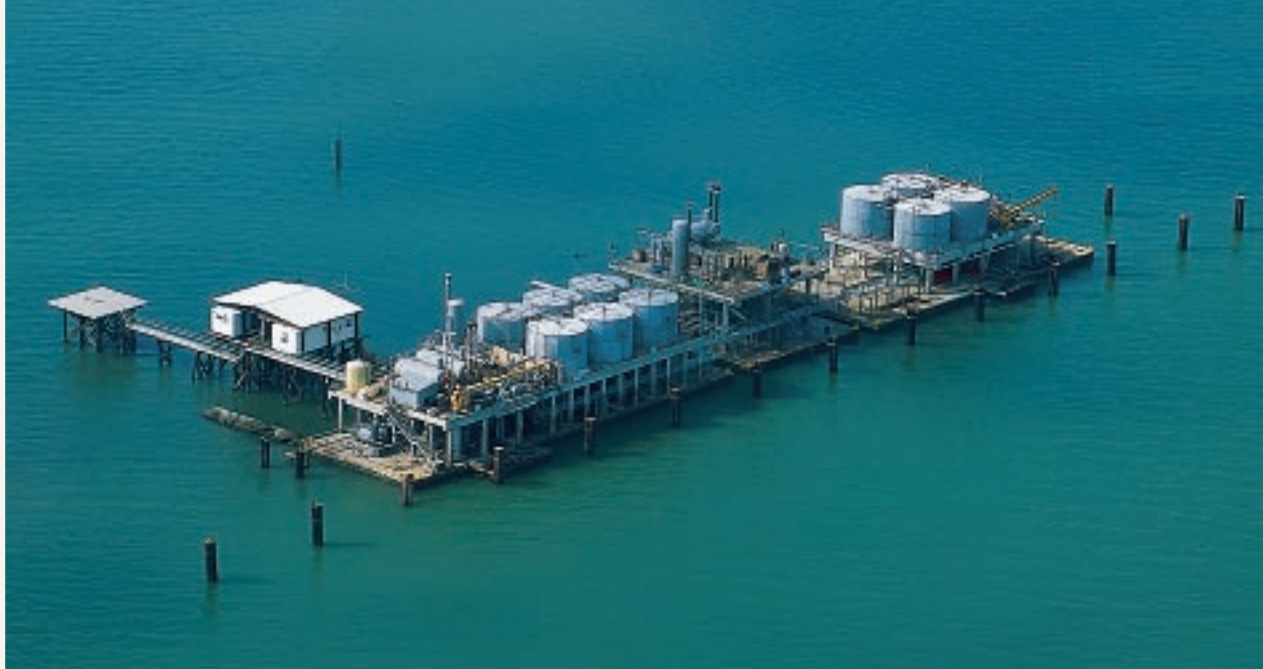
Central production and storage facility for the Ship Shoal/South Pelto area
